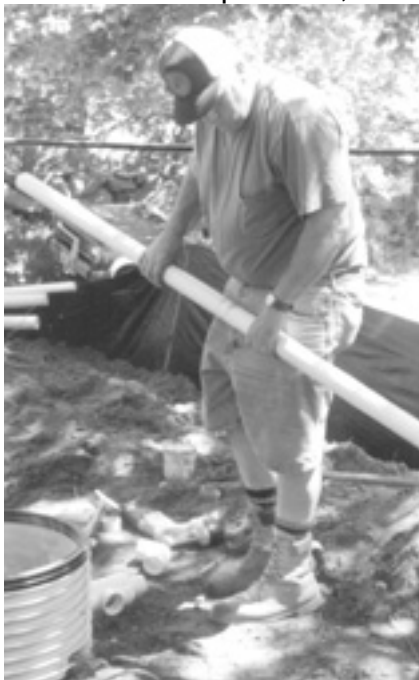
David Burnham, R.I. Independent Contractors and Associates president, installs piping for an alternative septic system at a demonstration site on Block Island. Photo by Monica Allard Cox.
